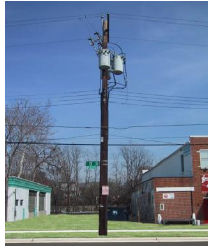
Figure 1B: Utility pole (Overhead System)
